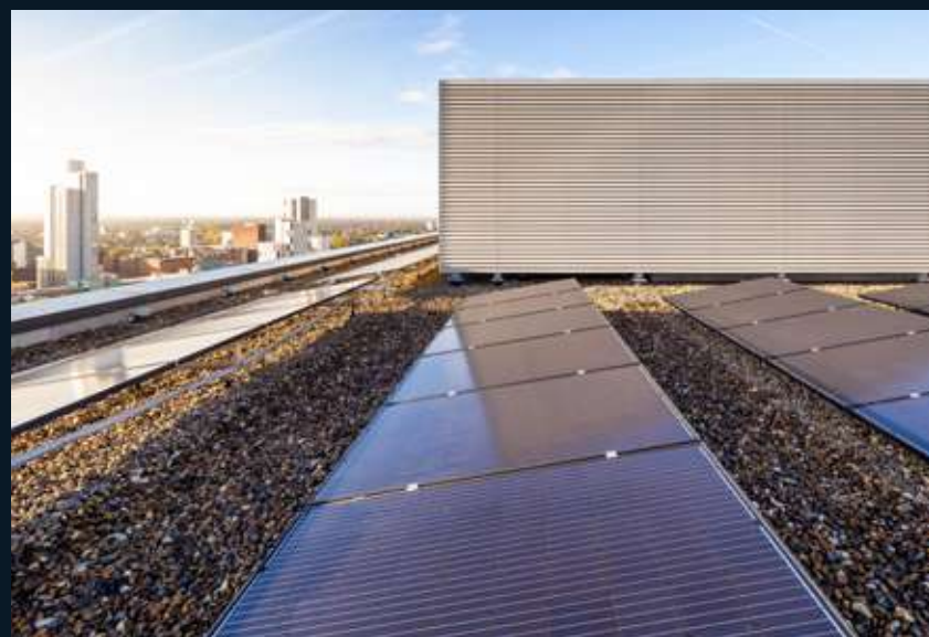
Landmark rooftop solar panels
