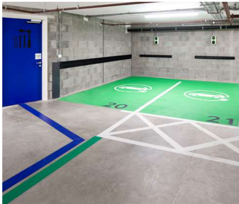
Electric car charging points
